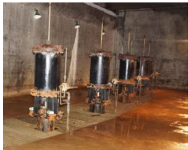
Shaft 7 valve actuators
