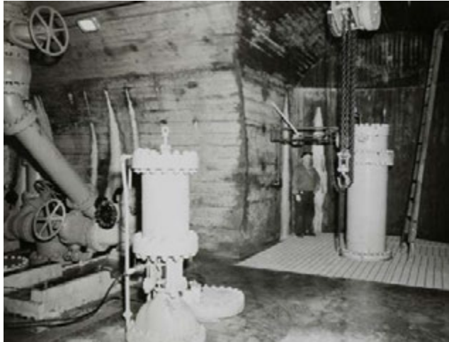
1959 photo of valves in Shaft 9 Chamber
