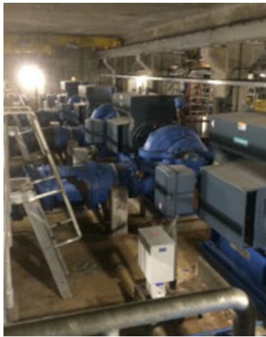
Chestnut Hill Emergency Pump Station
