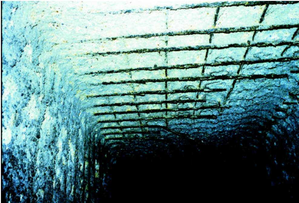
Photo #34: Section 137 Drop Chamber - Top of roof slab 20 feet below New Haven Street - Significant deterioration of 18 - inch roof slab. Steel reinforcing severely compromised.
