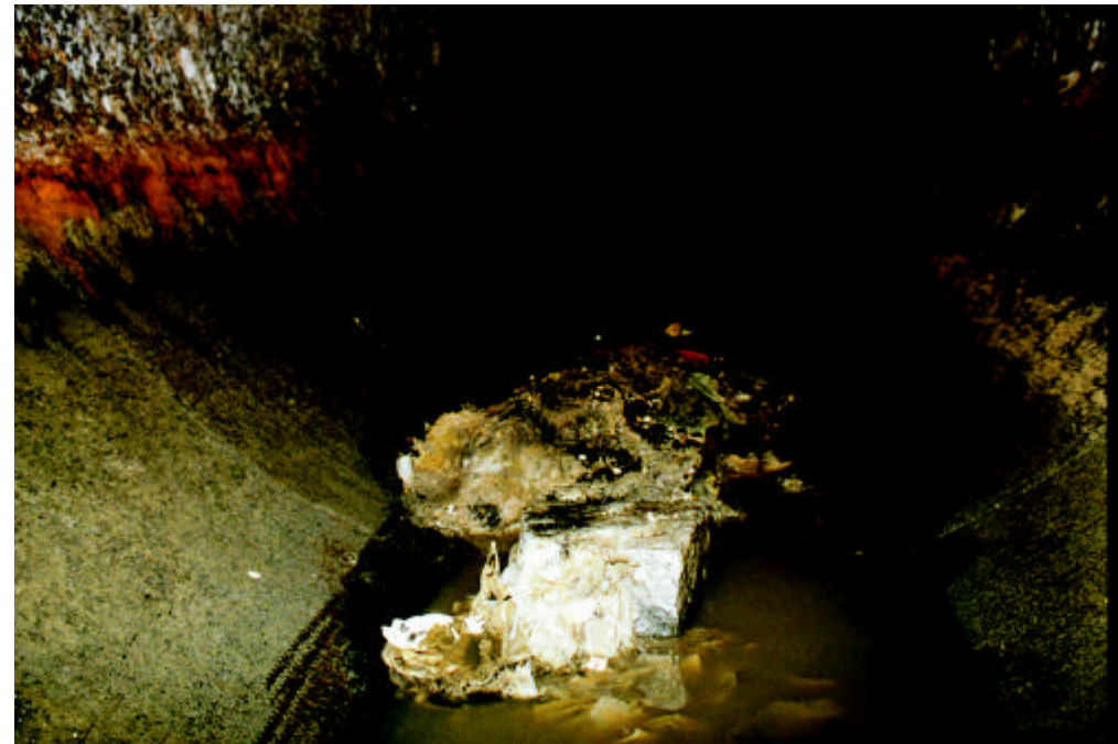
Photo #13: Section 138, station 198+63, 7-foot diameter sewer, West Roxbury-Below McDonalds parking lot. Top of pipe 17 - feet below surface. Debris at sewer invert. Corrosion above water line.
