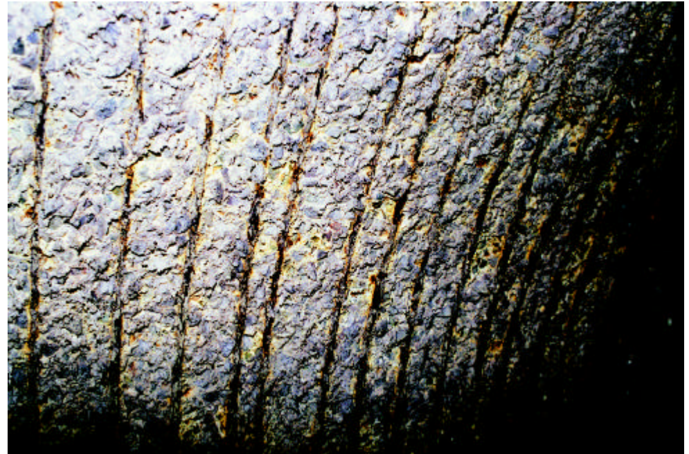
Photo #07: Section 138, station 200+88, 7-foot diameter sewer, West Roxbury-Open space behind McDonalds parking lot. Top of pipe 12 - feet below ground. Significant deterioration of concrete and steel reinforcing.
