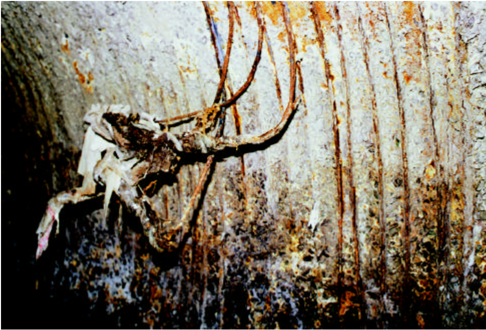
Photo #06: Section 138, station 200+60, 7-foot diameter sewer, West Roxbury - Open space behind McDonalds parking lot. Top of pipe 12 feet below ground. Photo shows significant deterioration of concrete. Reinforcing steel completely compromised.
