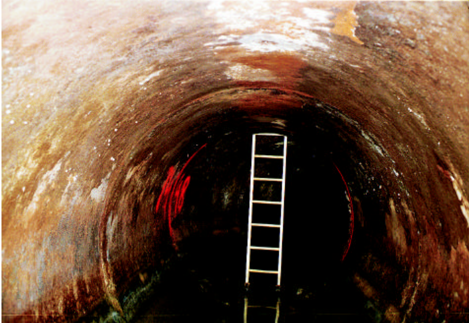
Photo #106: Section 137A, station 66+60, 7-foot diameter sewer, West Roxbury-East end of "West Roxbury Tunnel" Looking east toward Grew Avenue. Top of Pipe 17 feet below ground. Very good condition. No significant corrosion present.
