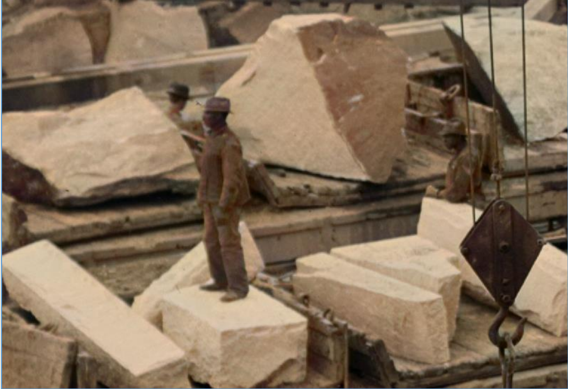
Chaining the huge rubble stones on flatcars for delivery by cableway to the work below.
